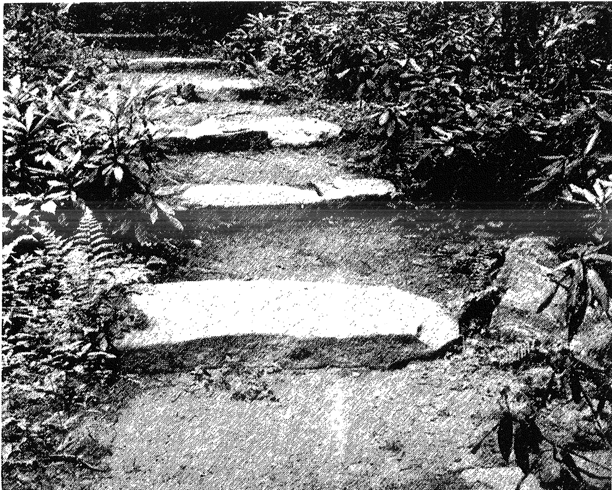
Rustic Stone Steps, Bronx River Parkway. These steps are cross-pitched to remove surface water flow off of trail.
